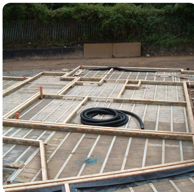
Figure 1: Sole plates laid out on masonry upstands above a beam and block floor
