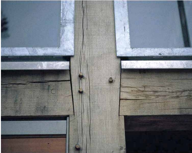
Figure 5: Traditional carpentry joint in a modern green oak structure Photo: Peter Clegg/Feilden Clegg Bradley Studios
